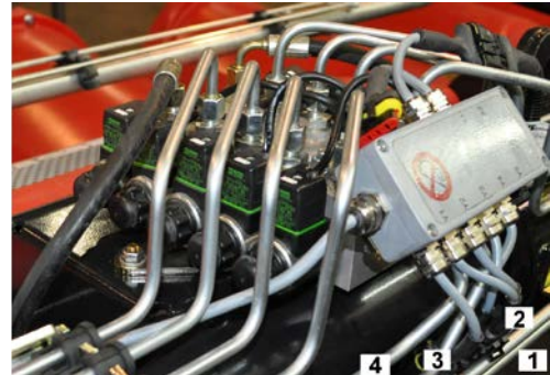
Central hydraulic system
