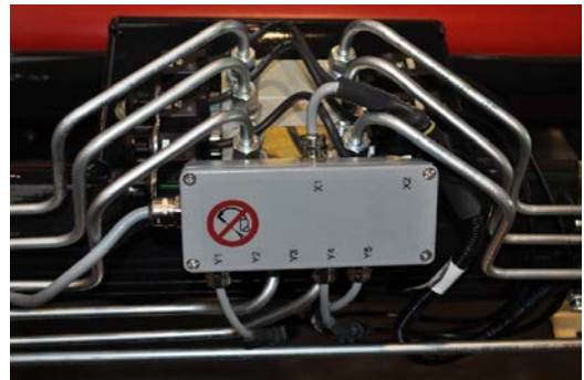
Central hydraulic system
